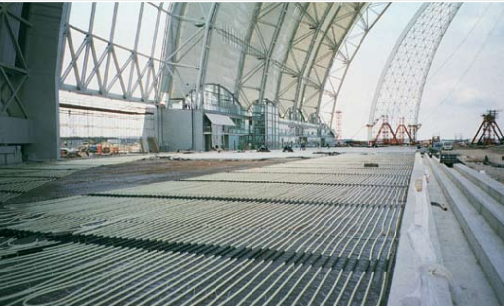
Roth Pipe Holder Component System, Tropical Island, Krausnick-Groß Wasserburg, Germany
