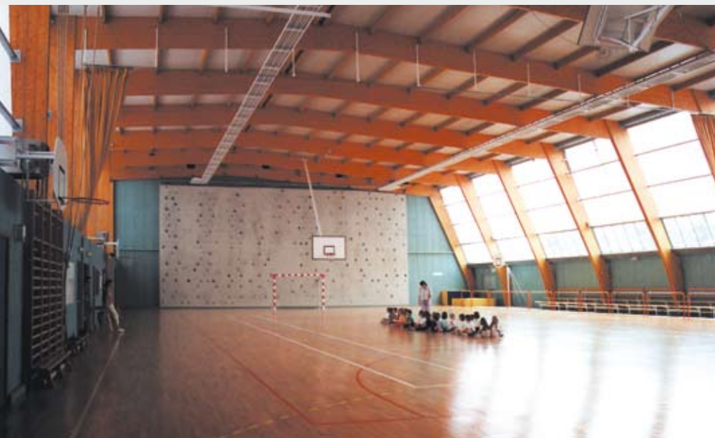
Roth underfloor heating, sports hall and fitness centre, Barbezieux, France
