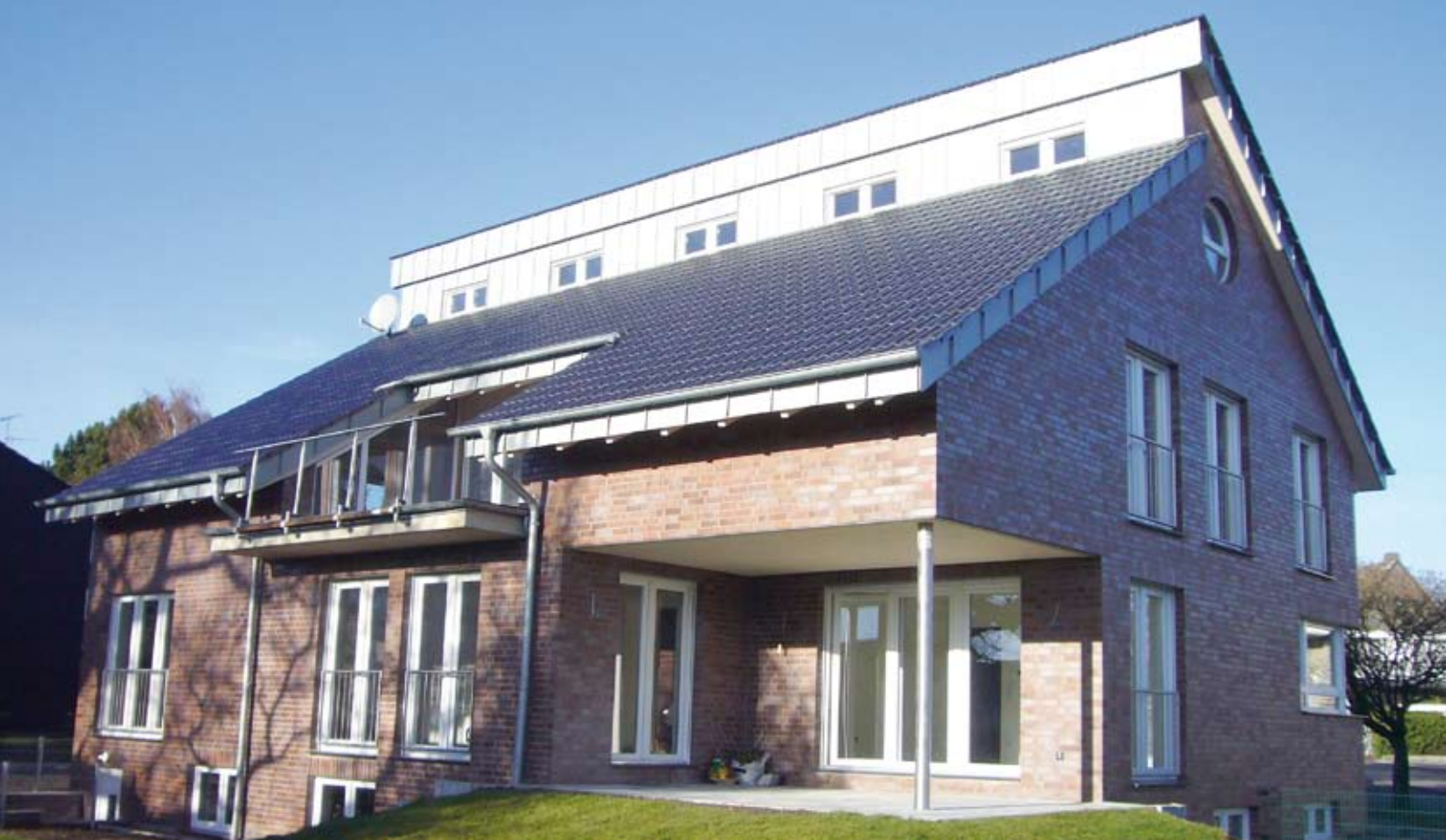
Roth underfloor heating (Roth Original Tacker® System with 17 mm X-PERT S5®+), Roth TerraCompact® 17 kW heat pump and Roth DUO impotable water storage tank 500, family home, Oer-Erkenschwick, Germany
