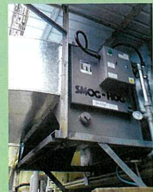
SMOG-HOG Electrostatic Precipitator installed at Cafe de Coral 大家樂內的靜電除油煙器
