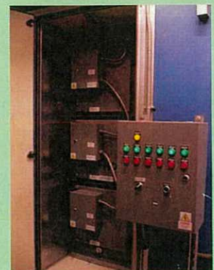
SMOG-HOG Electrostatic Precipitator installed at Shek Wu Hui Market 石湖墟街市內的靜電除油煙器
